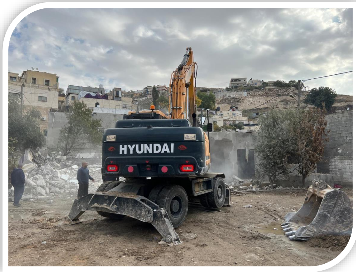
During the implementation of a forced self-demolition order for the Nassar family in the Wad Qaddoum neighborhood in Silwan town
